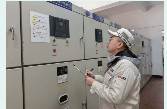
Employee monitoring power supply system operation data
