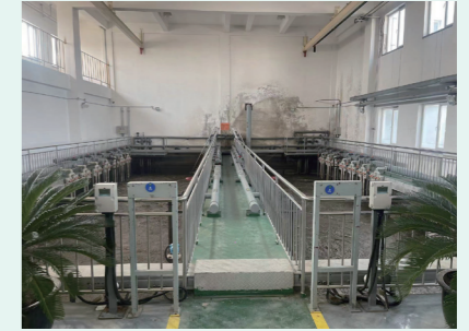
Reclaimed Water Reuse Equipment
